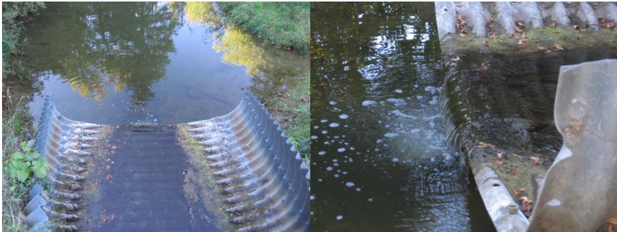
Above: Culvert that is blocking fish passage at the outlet of Spring Lake in Lengby.
