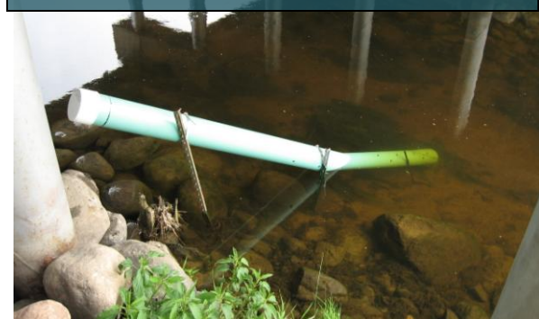
Site 757 (Mud River) Water Quality & Level Logging Station
