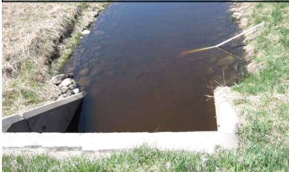
Stream Gauge 6 on Ditch 200 Water Level Logging Station
